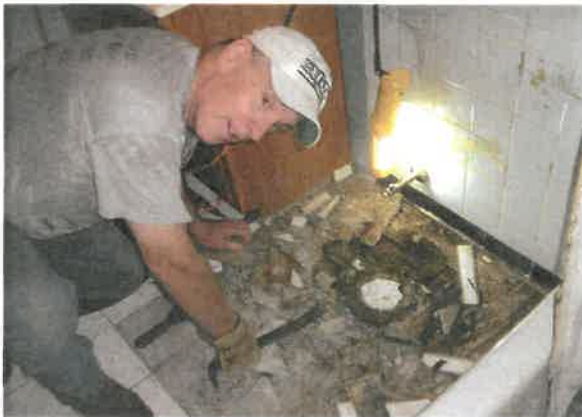
Pictured left: Our volunteer, Bob Campbell, repairing a plumbing leak in a client's bathroom.
