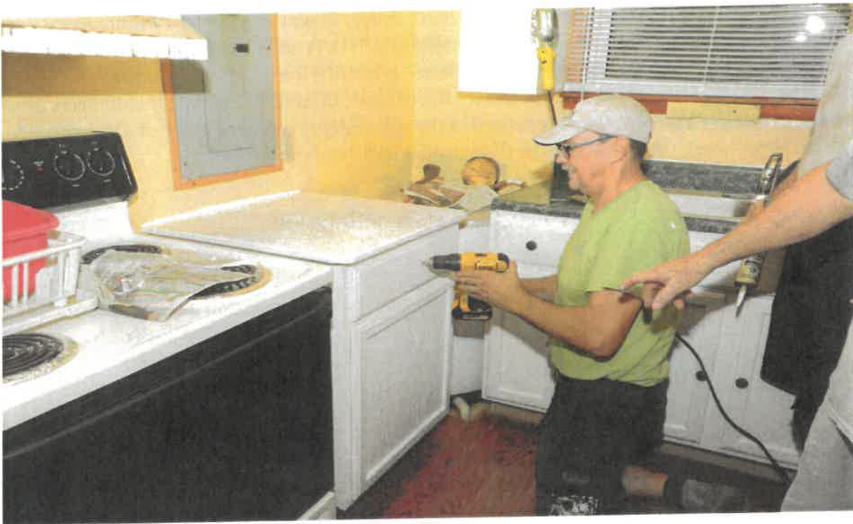
Volunteer Jim Overturf installing new kitchen cabinets for a client to replace those damaged by a water leak.
